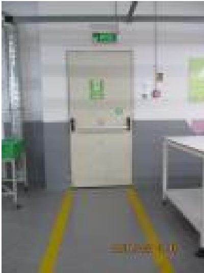
Emergency Exit Door.jpg
