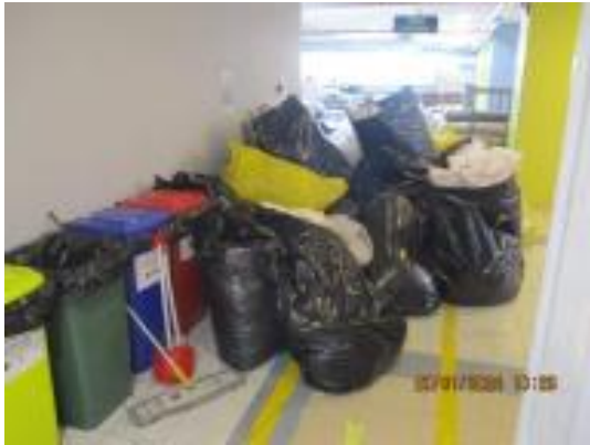
NC-Emergency Exit Route Blockage.jpg
